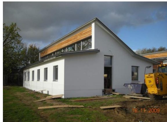
Undergoing Passive House certification – the new building for Disability Essex. Pictures courtesy of Simmonds Mills
